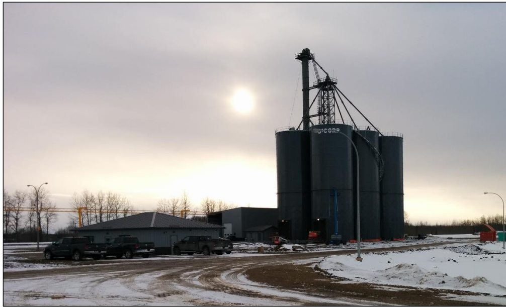
Photograph No. 3: Photograph showing the completed construction of the silos on the 700 m 3 slab.
